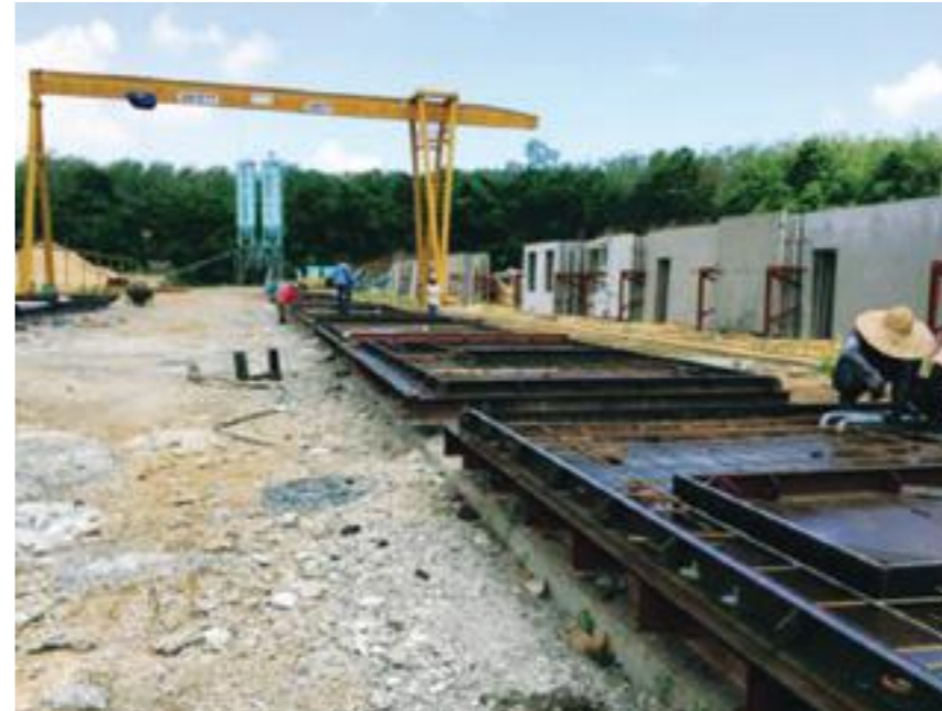
The components are produced at the IBS factory, where they undergo standardised manufacturing processes to ensure that stringent quality levels are met.
