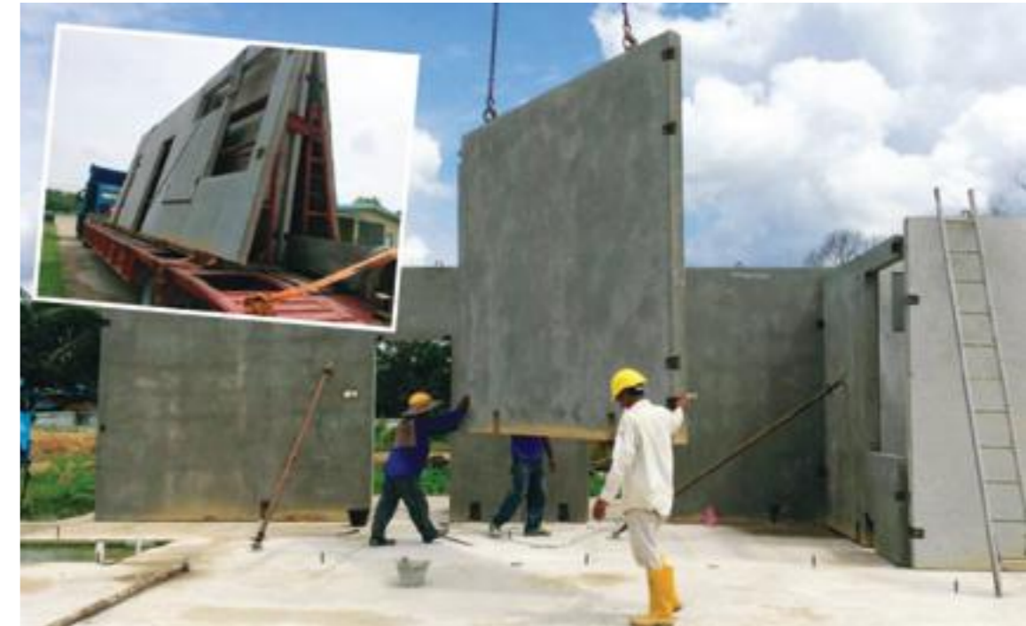
▲ After the panels have been manufactured at the factory, they are transported to the project site (inset) and installed.
