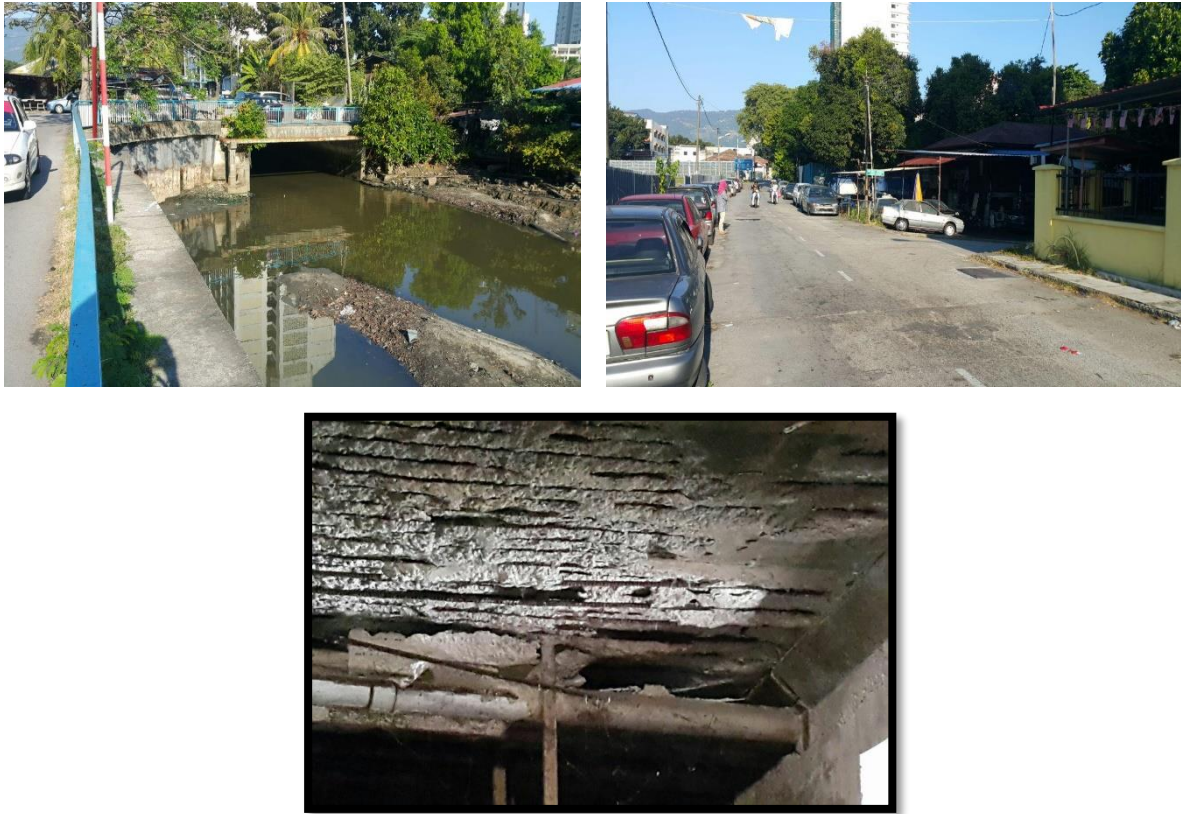
Figure 2.24: (left) Outlet of Sungai Jelutong Diversion (right) Top of Sungai Jelutong Diversion, Jalan Tengku (bottom) Inside the Sungai Jelutong Diversion before it is currently being rehabilitated
