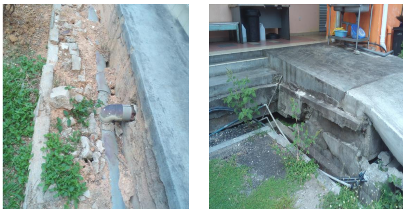
Fig. 1. Damage to the existing drainage system due to soil settlement at Politeknik Sultan Idris Shah, Sabak Bernam, Selangor.
