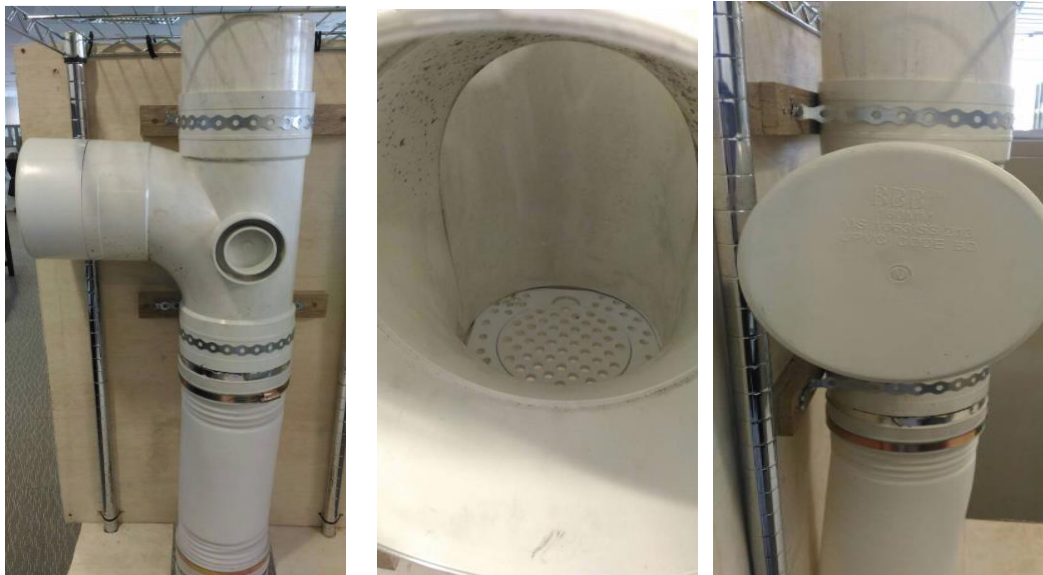
Fig. 7. Energy dissipator (strainer) installed in the rainwater down pipe
