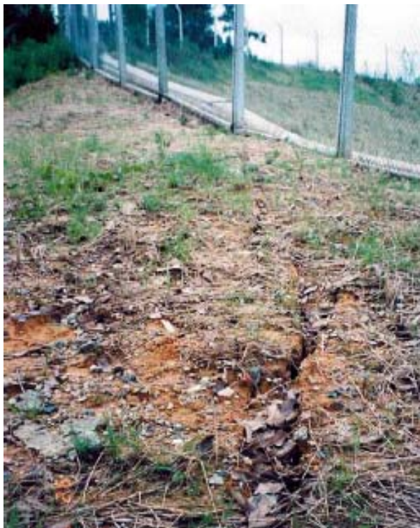
(a) Tension Crack on Slope
