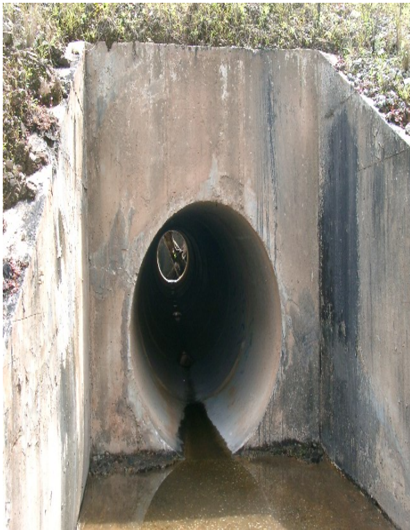
(c) Drain and Sump
