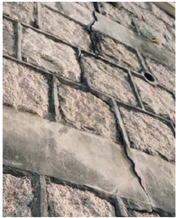
(b) Crack in Retaining Structure
